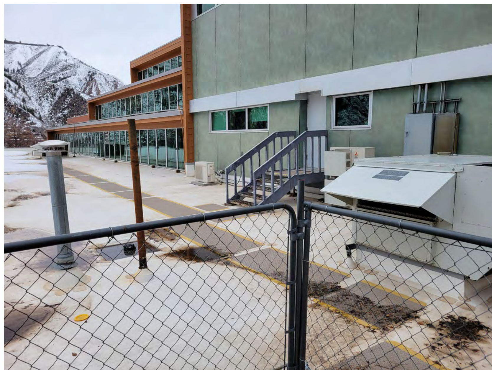
EXISTING ROOF CONDITION ABOVE MINI COLLEGE. SEE DRAWING FOR PHOTO LOCATION REFERENCE
