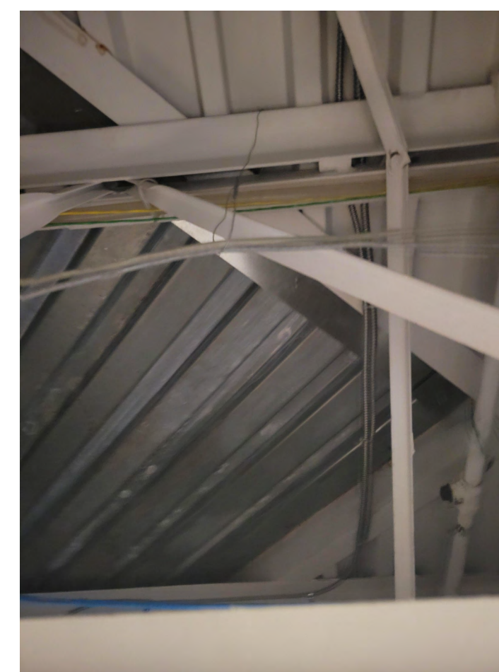
CORNER OF EXISTING SKYLIGHT OPENING - WHITE PAINTED DECKING & TRUSS TO STAY, DEMO SILVER DECKING CAP
